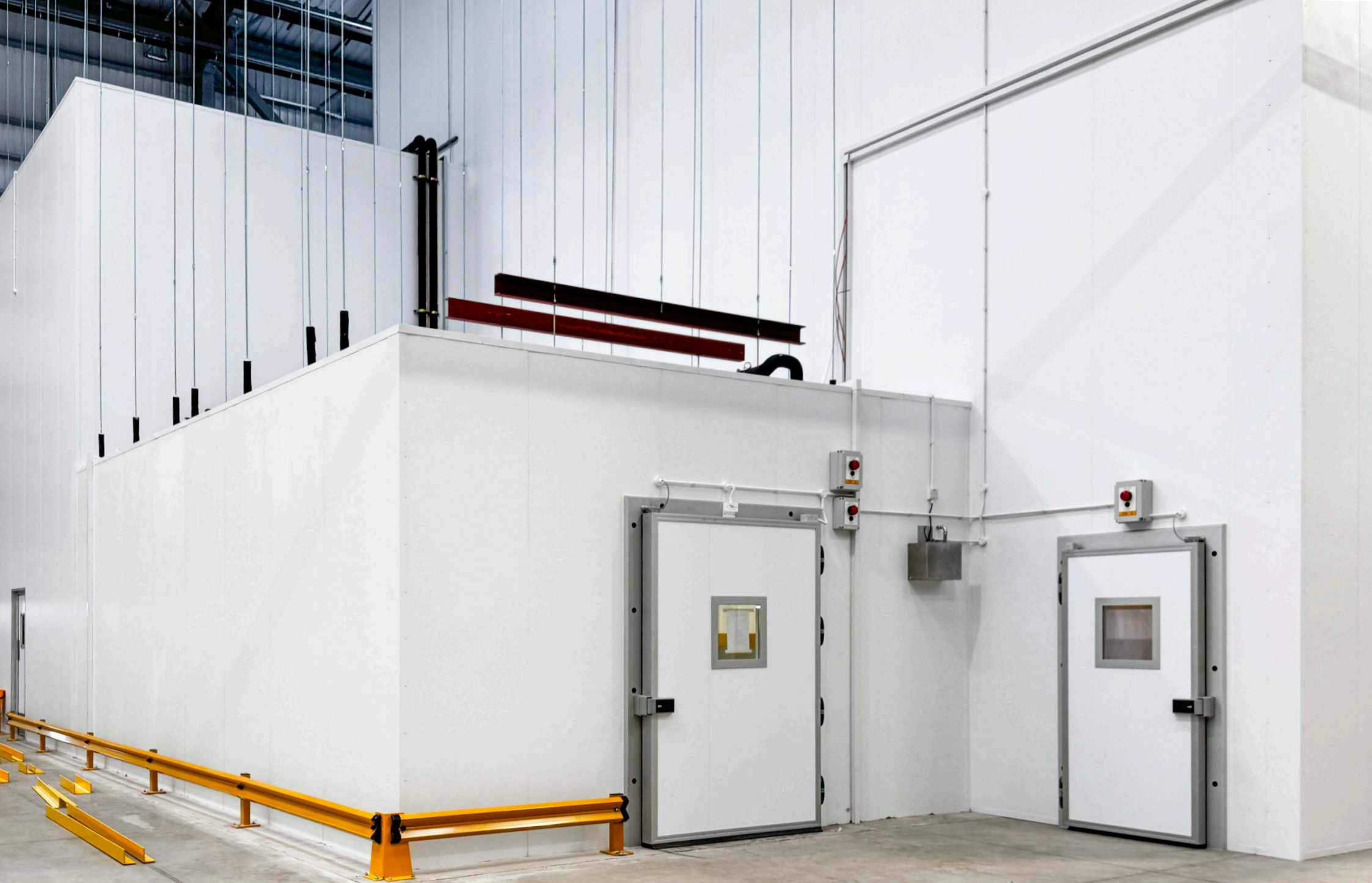
Freezer and Cold Room
